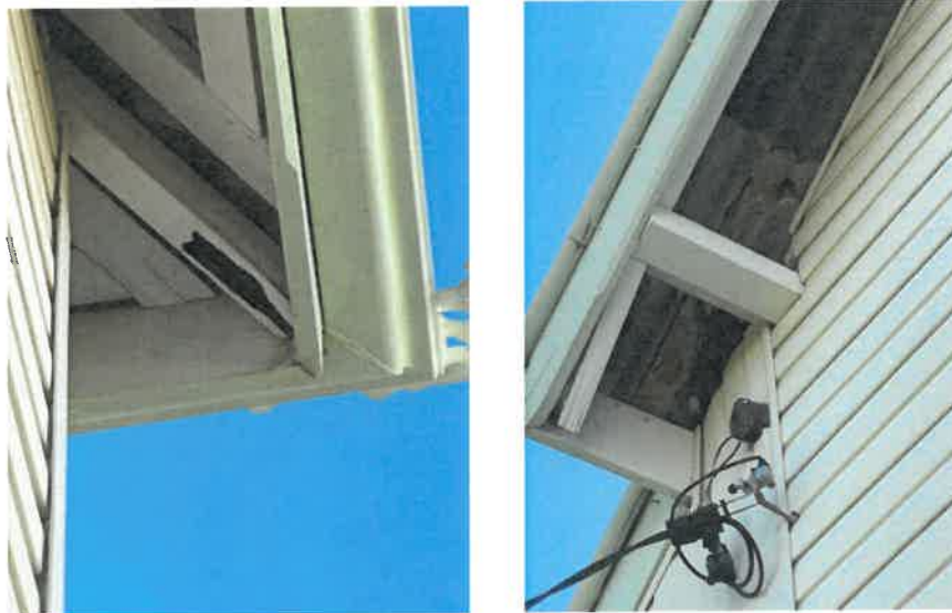
Figure 6: Deteriorated roof structure
